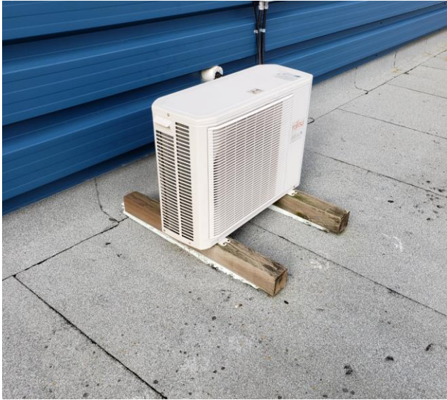
Figure 5: Additional Fujitsu split unit above multi-use area.
