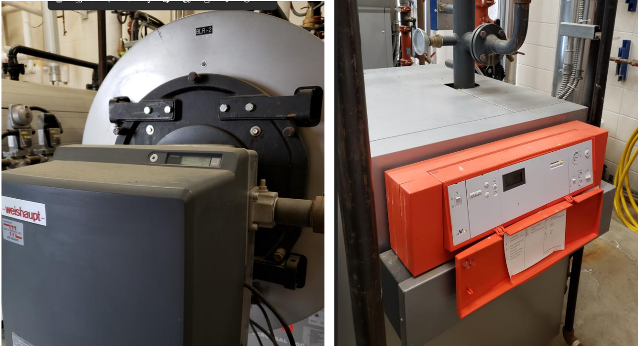
Figure 1: Boilers B-2 (left) and B-3. B-1 is the same make and model as B-2.
